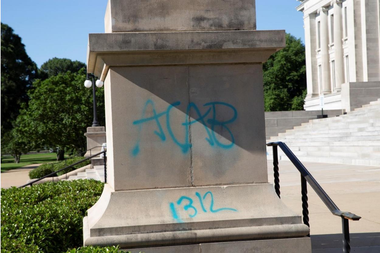
Photos of Damage to the Arkansas State Capitol Building, Lawn, and Surrounding Areas During the George Floyd Protests - Provided by AR State Capitol Police
