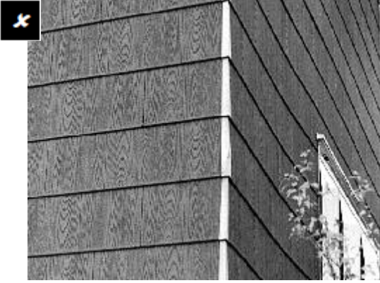
Imitation materials that are designed to look like wood or masonry siding, but that are fabricated from other materials, are inappropriate.
