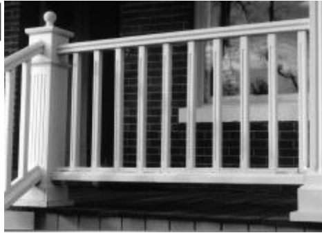
The spacing of balusters on this replacement railing is inaccurate.
