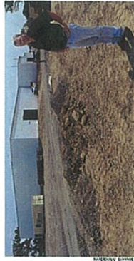
EDAMAME PLANT — Kelly Cartwright, AVS chief operating officer, supervises construction in Mulberry of the first U.S. facility for receiving, processing and packaging edamame vegetable soybeans on a commercial scale.
