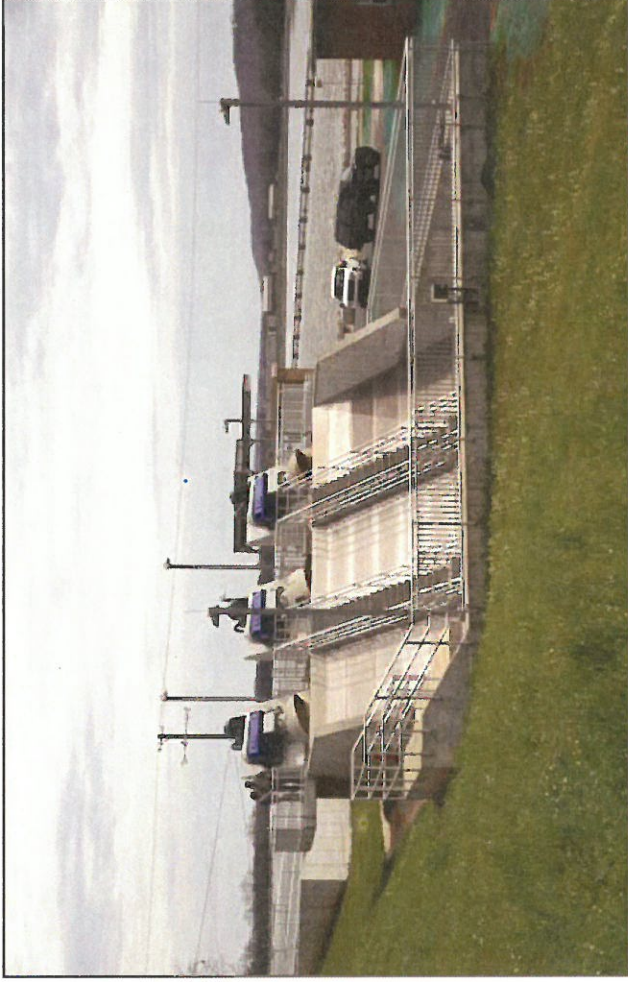
The 45 MGD screw pump lift station accommodates three 90-inch diameter screw pumps.
