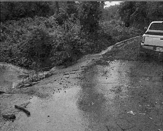
Roadside ditch delivers sediment runoff directly to the stream
