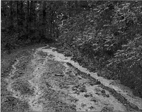
Runoff flows along the road, causing surface material to erode
