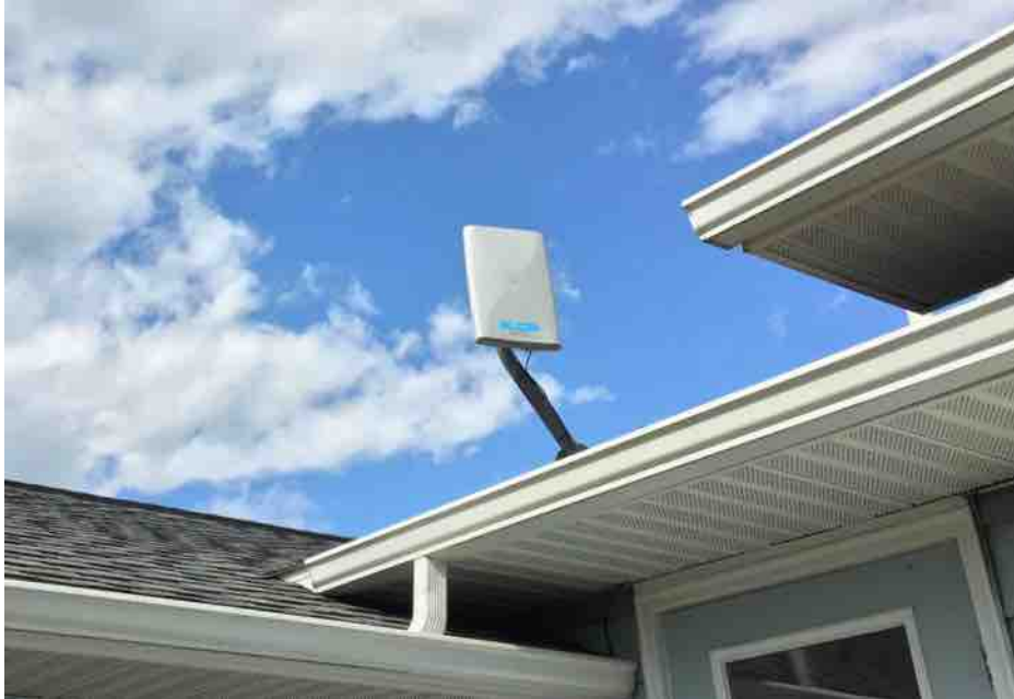
Figure 92. AT&T Fixed Wireless Device Mounted on Subscriber's Home
