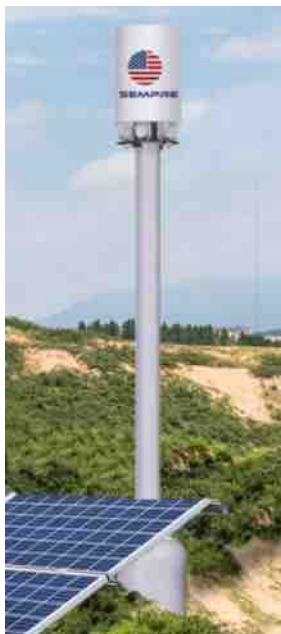
Figure 101. Sempre EMP-resistant tower and integrated edge data center
