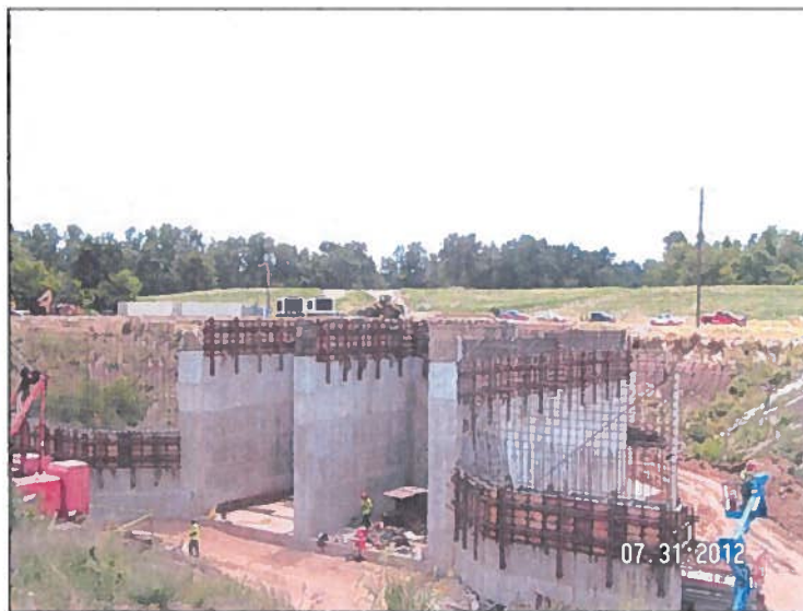
Little Bayou Metro Pump Station Construction is about 60 percent complete. Completion Date: December 2012
