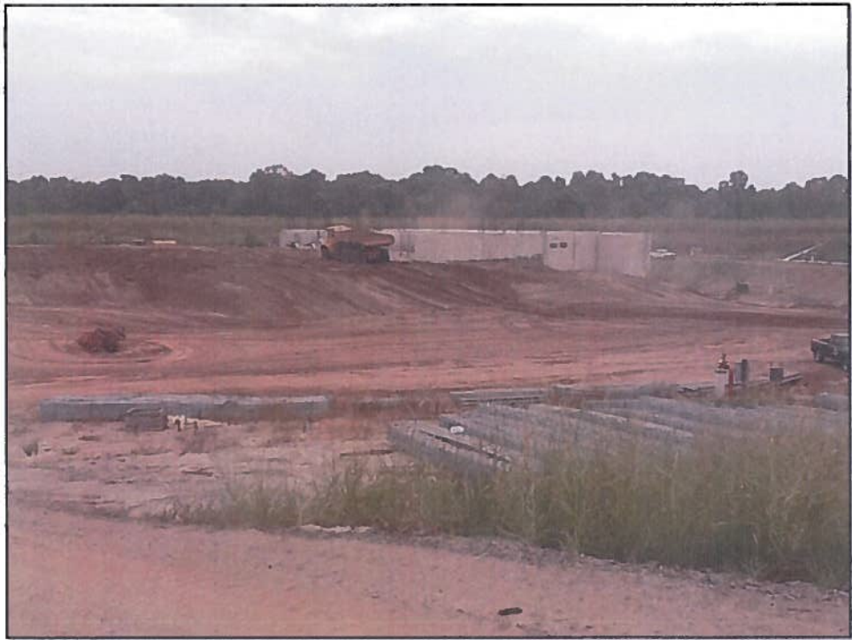
Grand Prairie Area Demonstration Project Pump station at DeValls Bluff currently under construction
