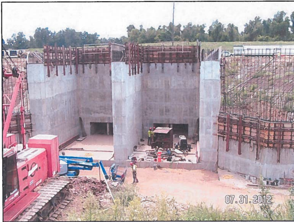
Little Bayou Meto Pump Station
