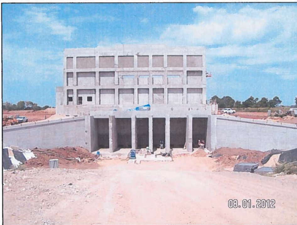
Bayou Meto Pump Station No. 1 inlet channel
