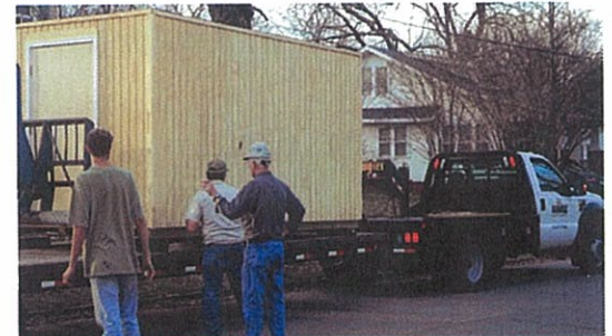
This apprentice class built two storage buildings and donated them to a local charity.
